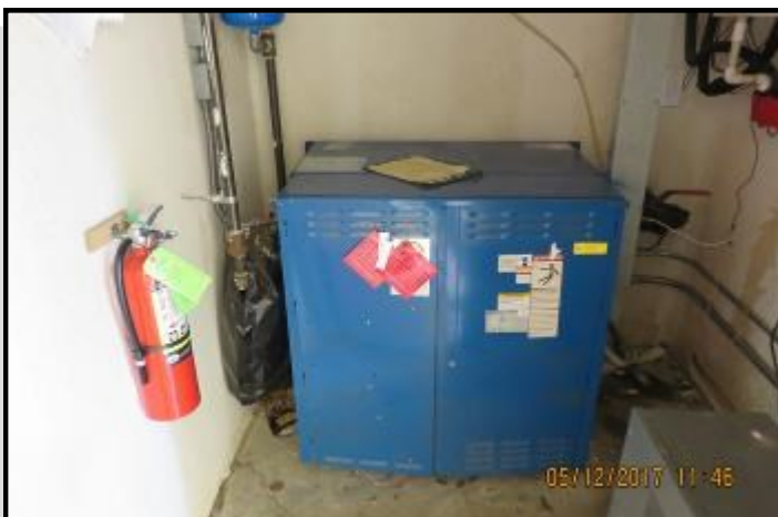
Hydraulic elevator equipment.
