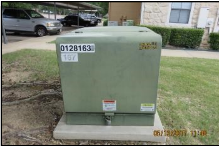
Pad-mounted electrical transformer.
