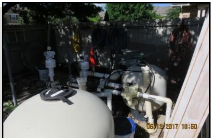
Pool pump and filtration equipment.
