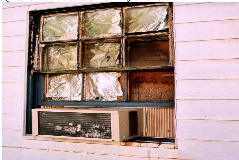
Weather damaged window in need of replacement.
