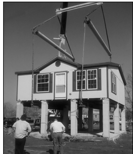
Above: Disaster recovery funds in Sabine Pass help to elevate a home to make it better able to weather future storms.
