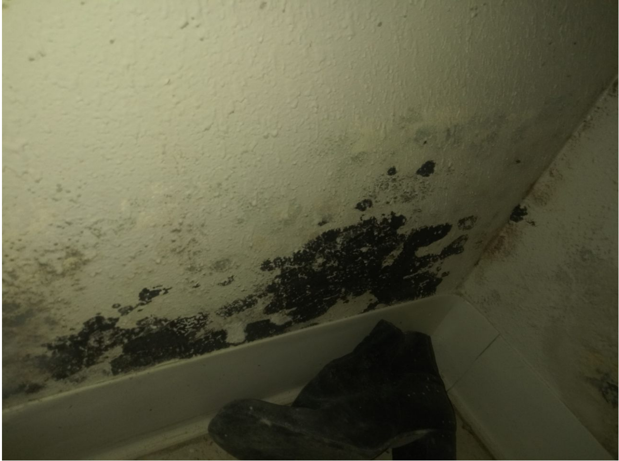
Sandpiper Cove Apartments – Water Damage and Mold on Walls
