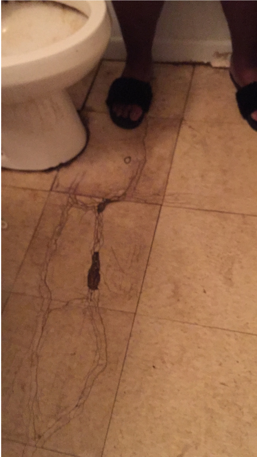
Sandpiper Cove Apartments – Mold and Damage to Floors
