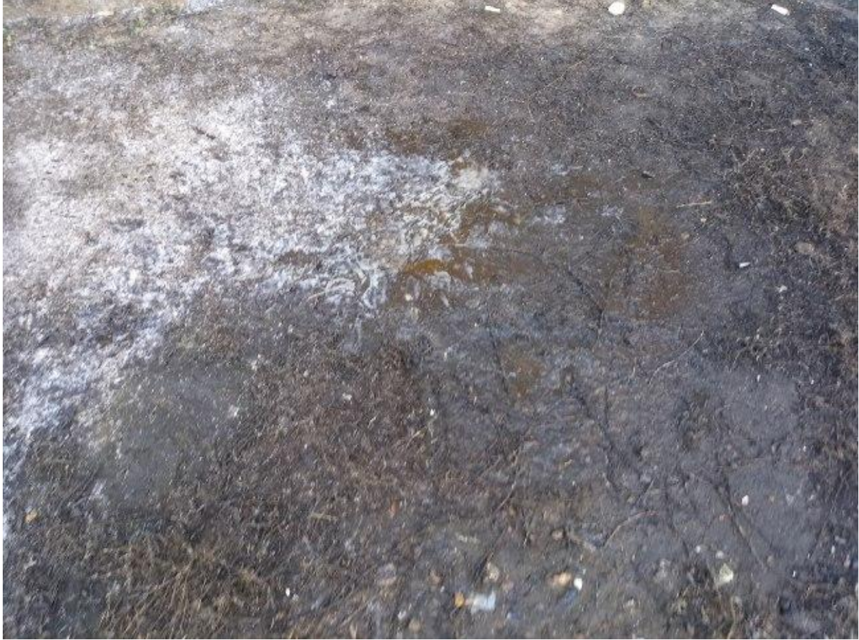
Sandpiper Cove Apartments – Exterior Sewage Overflow
