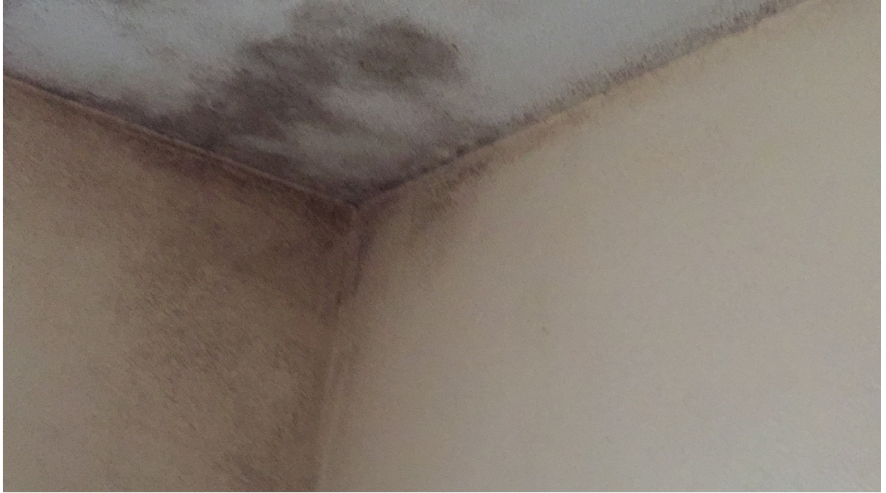
Sandpiper Cove Apartments – Mold on Walls and Ceilings
