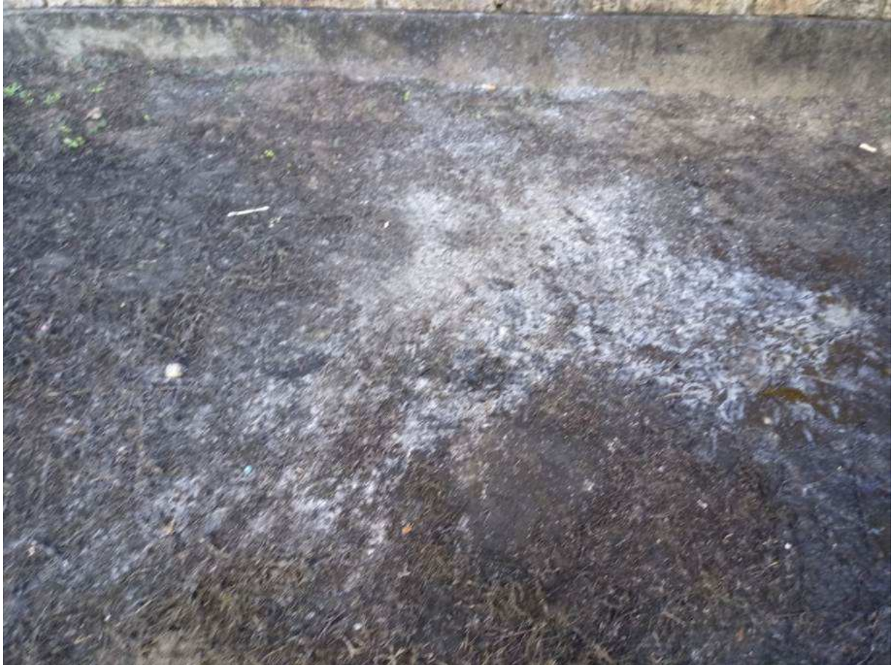
Sandpiper Cove Apartments – Exterior Sewage Overflow
