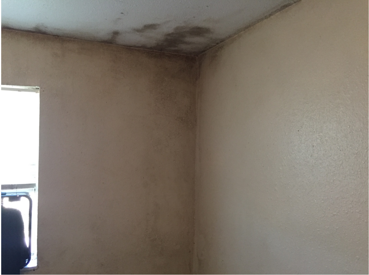
Sandpiper Cove Apartments – Mold on Walls and Ceilings
