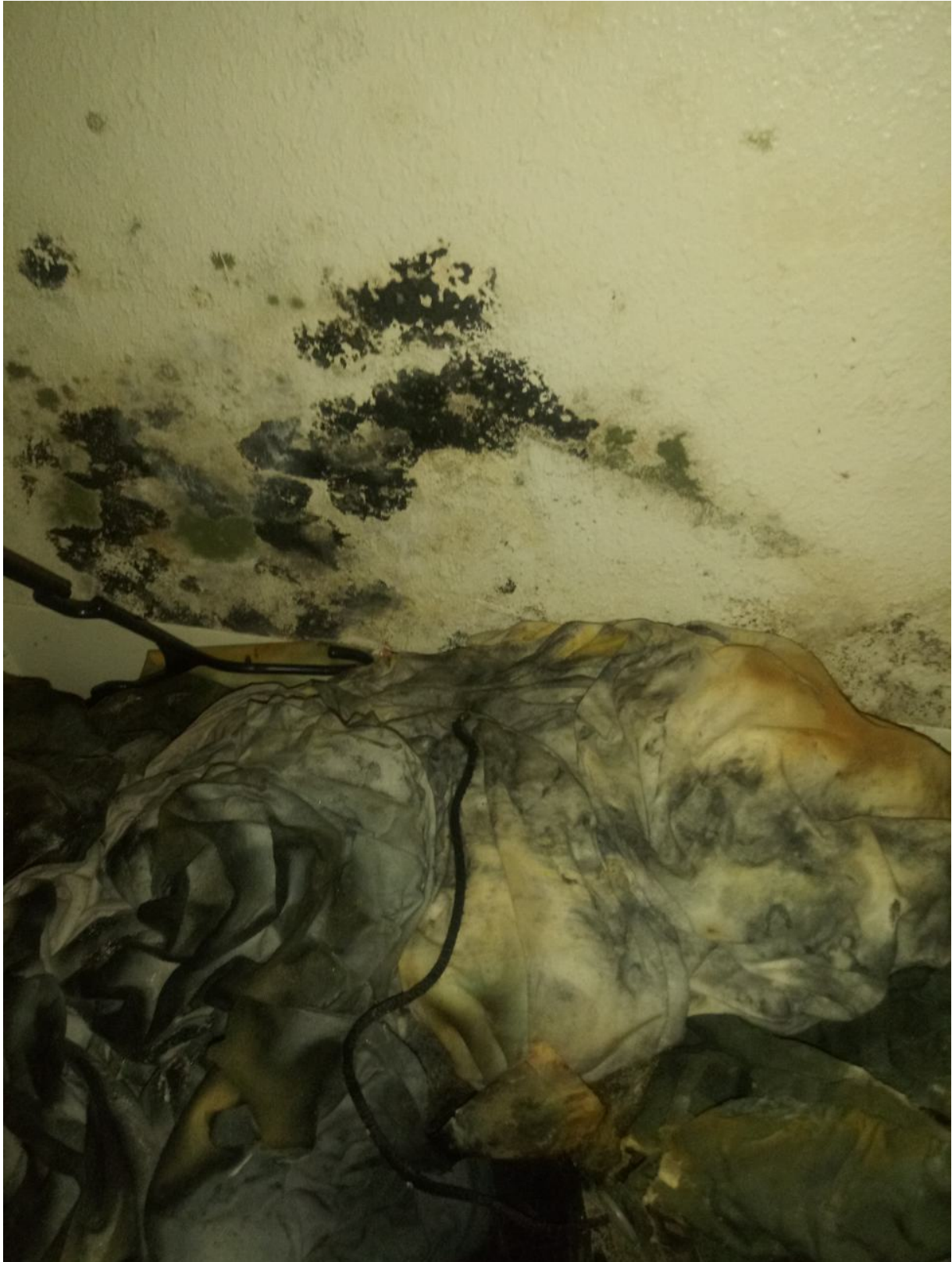
Sandpiper Cove Apartments – Mold and Water Damage in Elderly Woman’s Apartment
