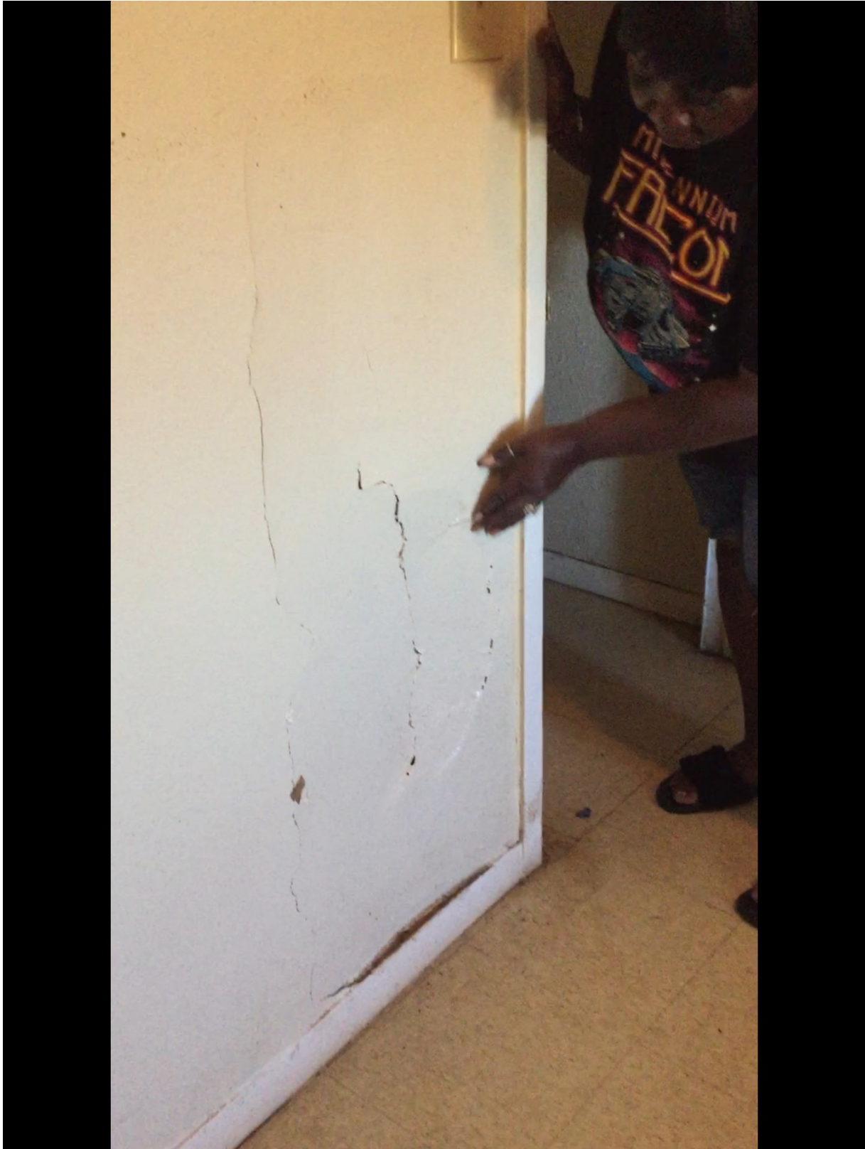
Sandpiper Cove Apartments – Water Damage to Walls
