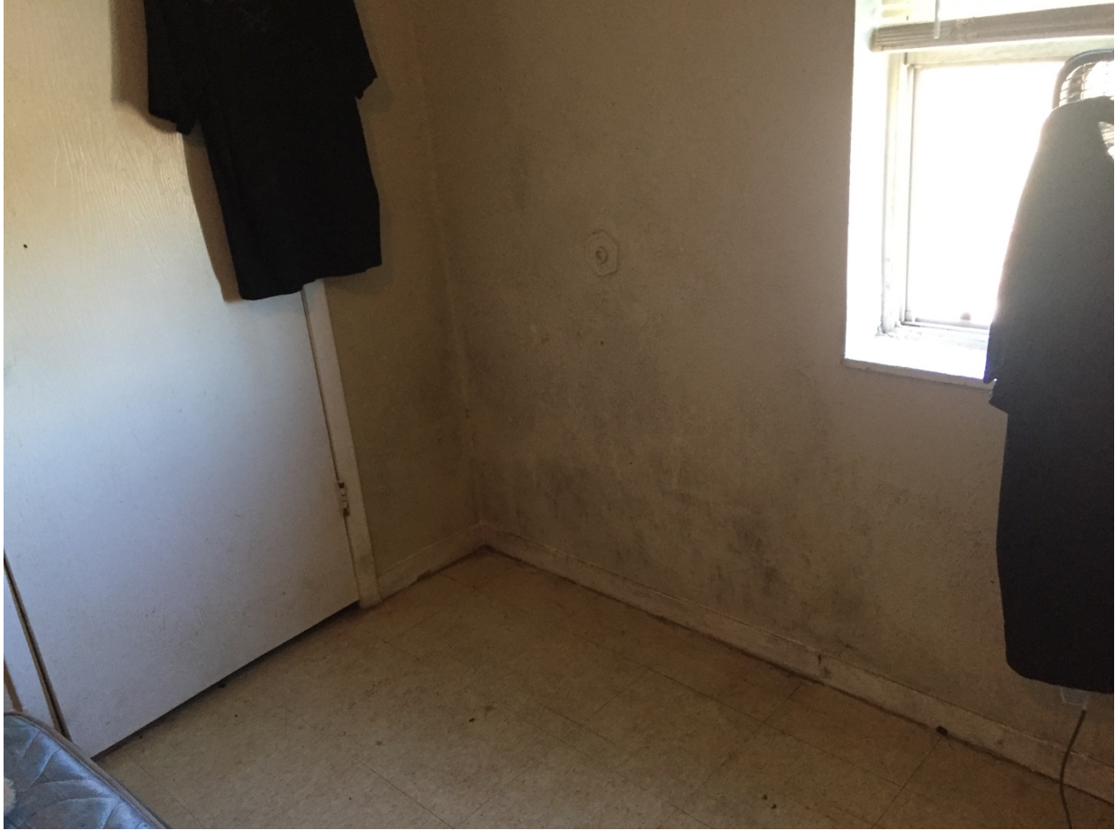
Sandpiper Cove Apartments – Mold on Walls and Floors
