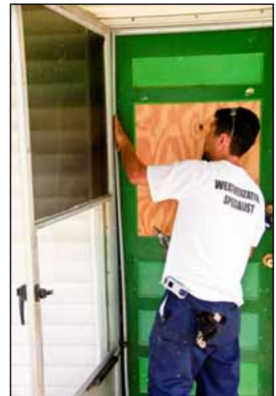
Above: A weatherization specialist with Houston's Sheltering Arms, funded through TDHCA's Weatherization Assistance Program, applies weather stripping to a low-income Texans' home.
