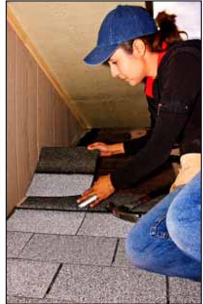
Above: A Texas Bootstrap Loan recipient places a roof shingle into place.
