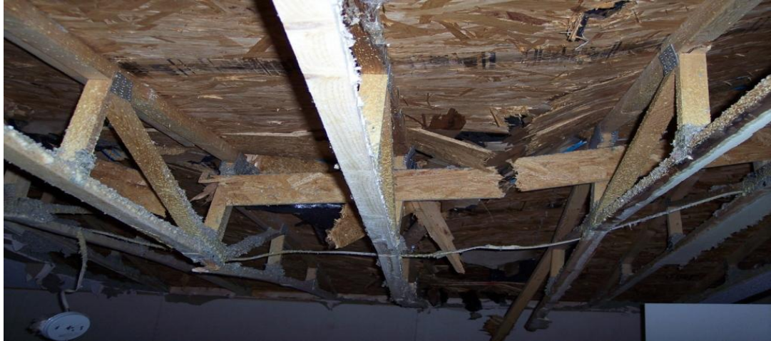
Figure 2 Interior view, current condition, shattered joists and rafters
