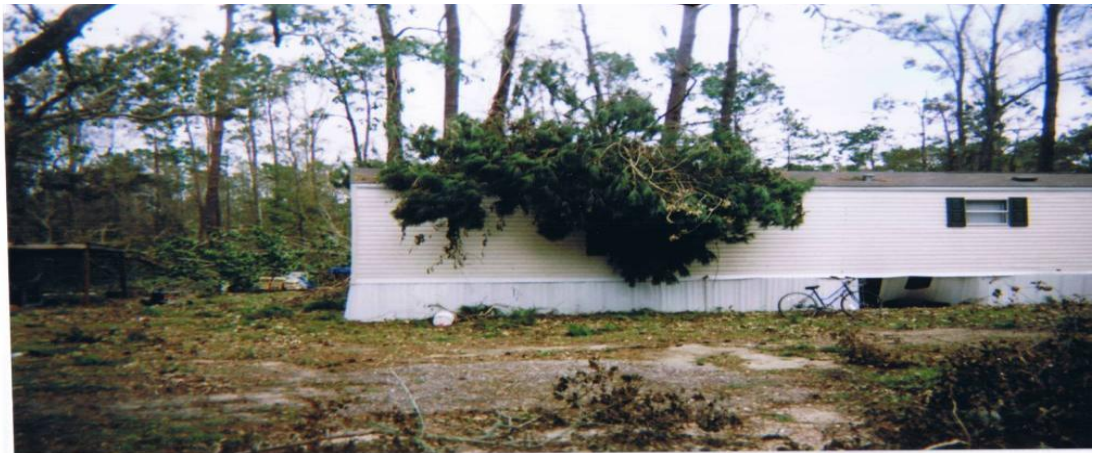
Figure 1 Uninsured manufactured home damaged by Hurricane Ike 6
