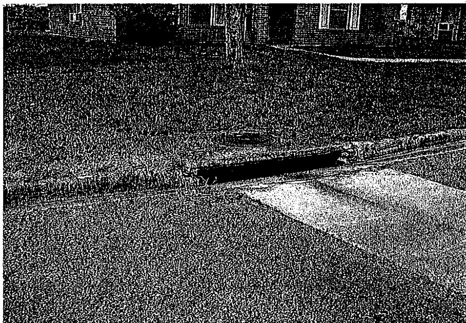
10. View of a typical curb inlet. Note: The concrete has cracked and the rebar is now visible.
