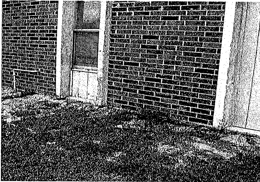
20. View of the soil erosion and rotted wood siding and trim boards.
