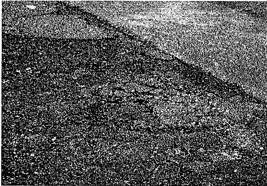
13. View of the raveled and extensively cracked asphalt pavement.
